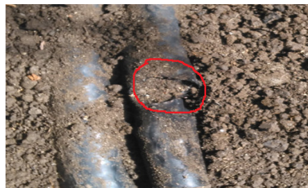
Fig.21. Visualization of the sleeve defect after the excavation
