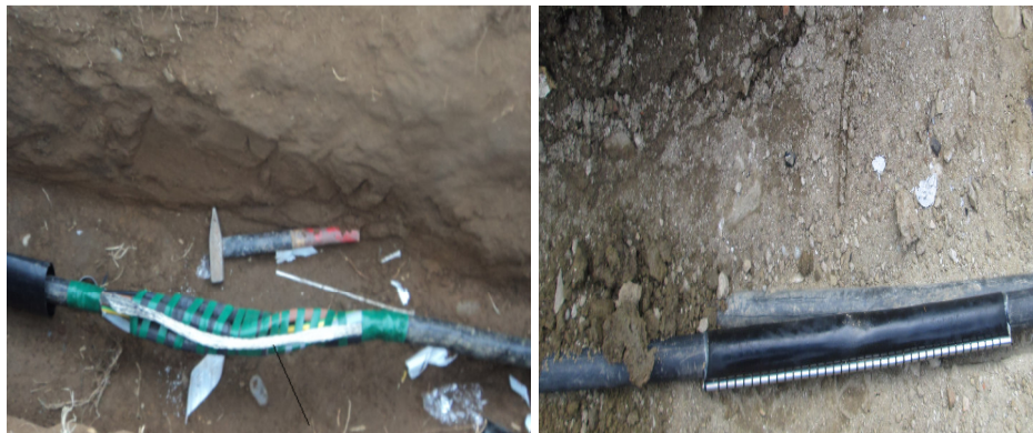
Fig.18. Installation of tinned braid with fixing rings for reinforcement transfer; Installation of the heat-shrinkable zipper sleeve
