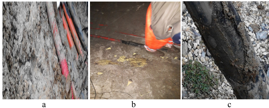
Fig.9.a),b). Identification of the sleeve defect on the solidified tailings portion c) The insulating (decomposed) portion of the heat-shrinkable sleeve resulting from the acid effect.
