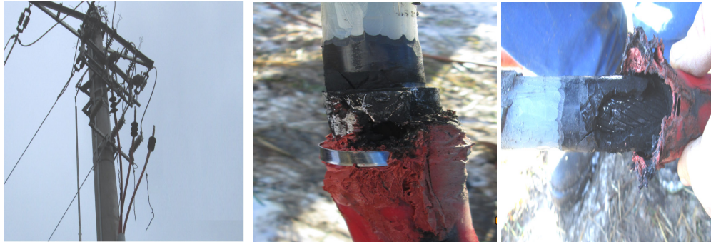
Fig.22. a) Detaching the copper shields from the earthing belt of the OHL pole and identifying the terminal head defect; b) Removing the outer shell and overviewing the defect.
