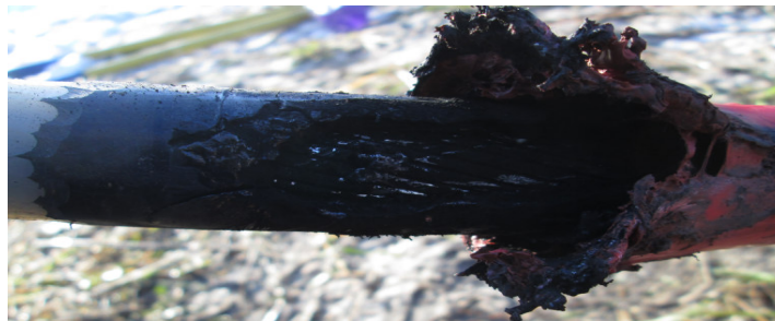
Fig.3. Insulation breakdown in the terminal head area [16]
