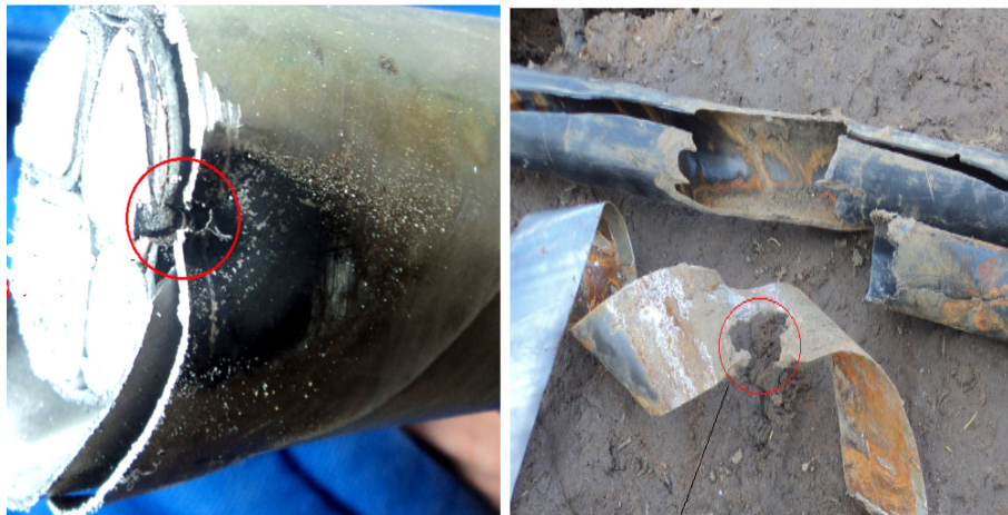
Fig.19. The point of insulation breakdown between the conductor and the metal reinforcement; The portion of the steel strip in which the electric arc generated the vibration phenomenon of the metal reinforcement.
