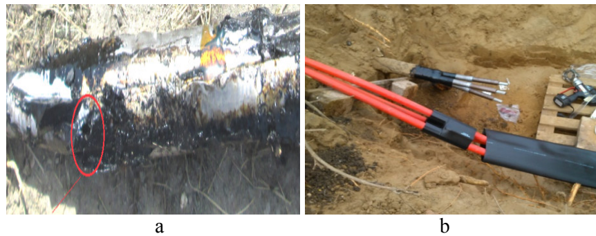
Fig.25 . a) Identification of the breakdown point in the cast iron jacket; b) Cable sleeve using two transition sleeves from HIU cable to three cables monopolar cables with XLPE insulation.
