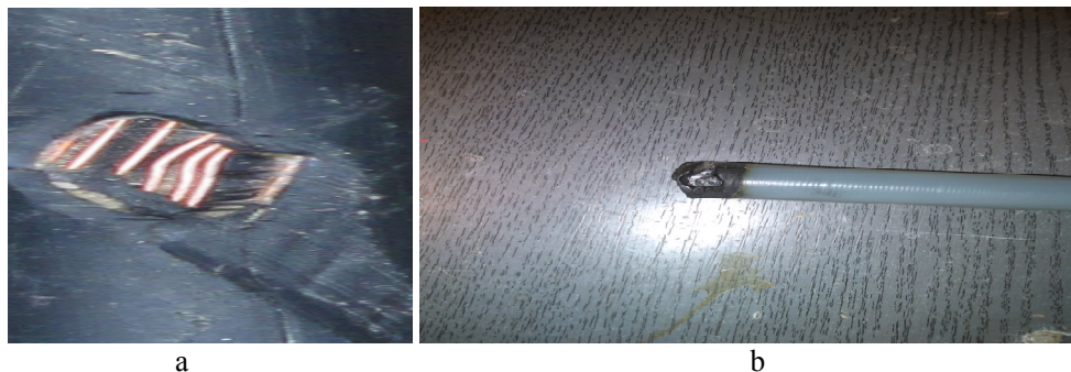
Fig.7. View of the insulation breakdown location :a) after removing the outer coating. b) after removing the semi-conducting layer
