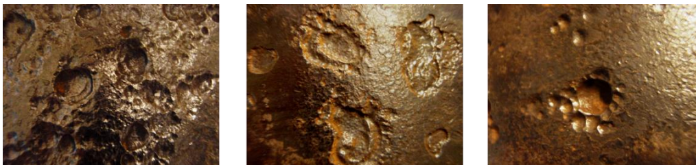
Fig.2 Pitting terasat specific coroziunii microbiologice
