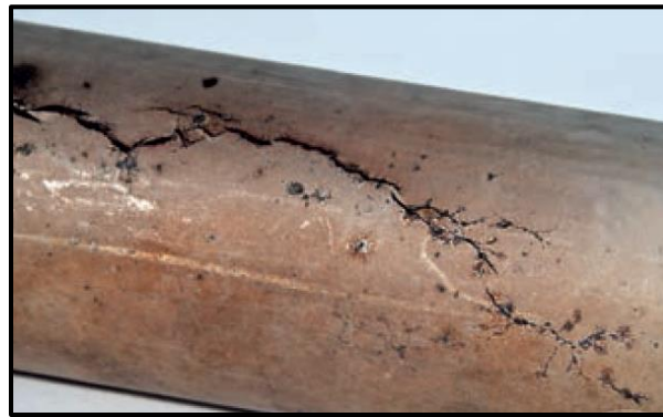
Fig. 3.1 Stress corrosion cracking for stainless steel tube [1]
