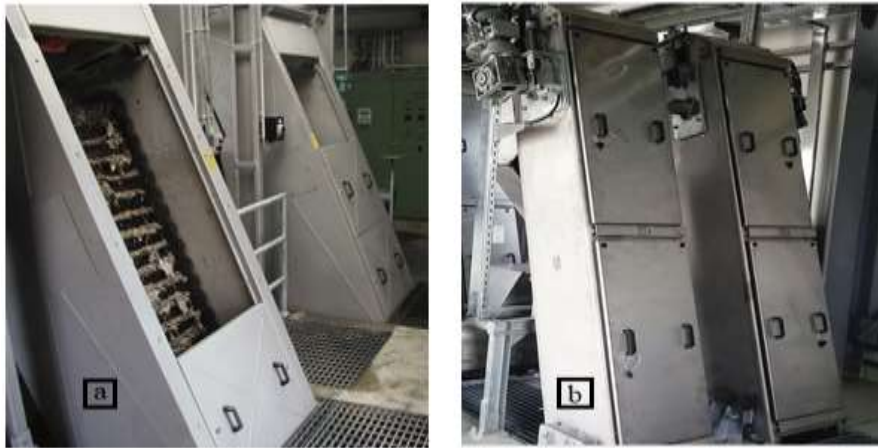
Fig. 6.65. Dense bar screens (a), respectively rare (b) from the structure of the urban wastewater treatment plant
