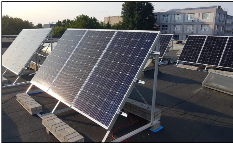
Figure 4.8.a Photovoltaic panels - component of the ICPE ACTEL SA photovoltaic power plant
