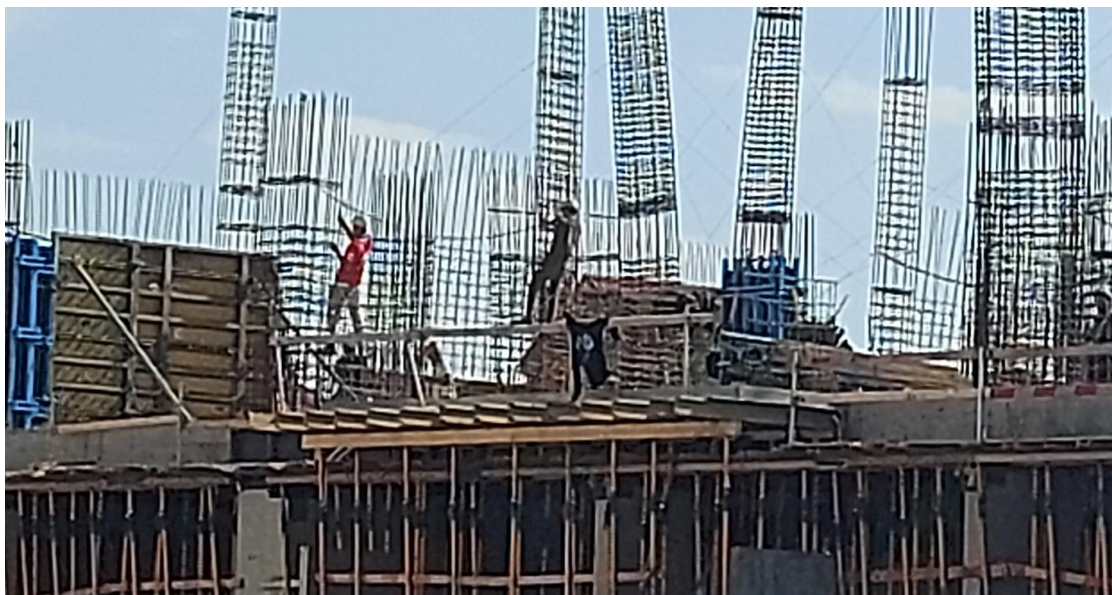
Picture 1.9. Lack of coordination, overlapped works, workers lacking the minimum individual workwear equipment
