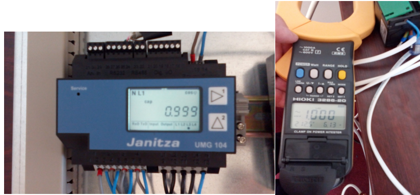
Indication of the numerical counter and the standard measuring meter
