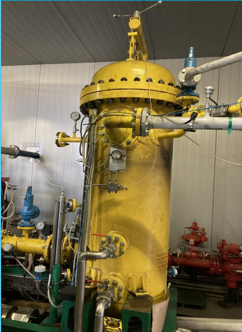
Figure 4.40. The instrumentation of DN800 PN50 separator vessel
