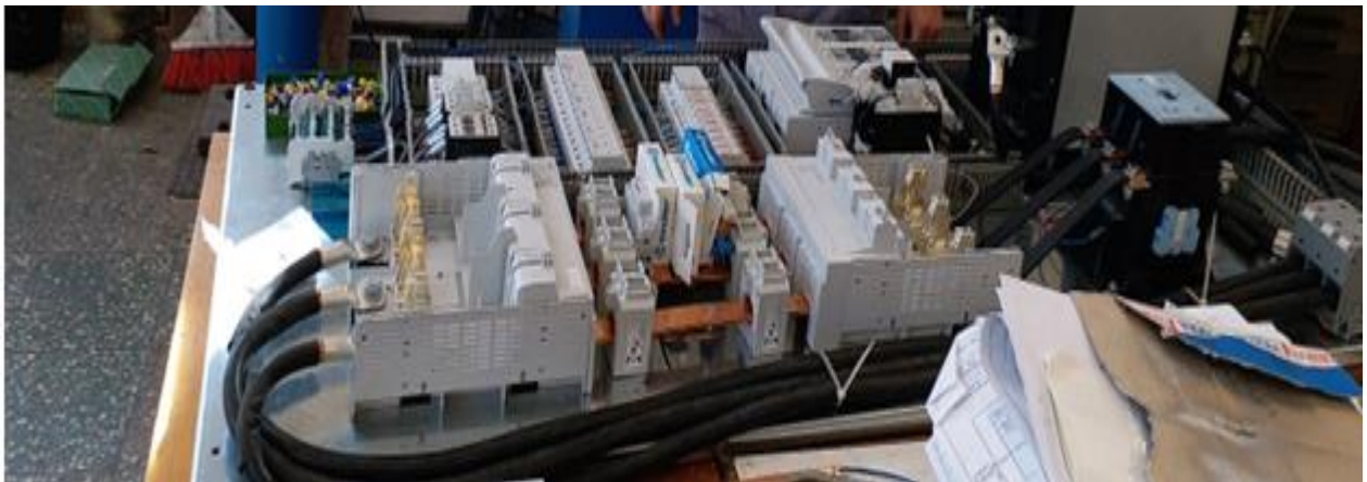
Fig. 12 – The ongoing execution of the power cabinet from the Electrical and Automation Engineering Laboratory at COMOTI
