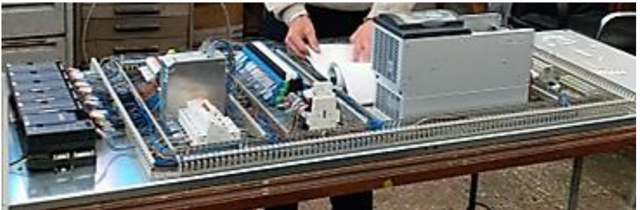
Fig. 13 – Execution of the automation cabinet in progress, from the Electrical and Automation Engineering laboratory at COMOTI
