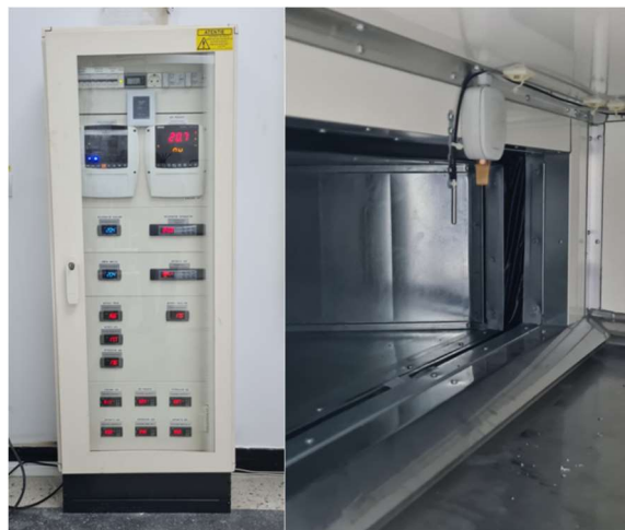
Fig. 3.5 The monitoring board of the air conditioning installation and the positioning of the sensors in the air handling unit
