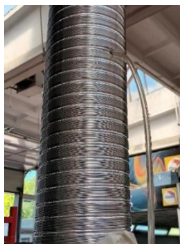
Fig. 19 Execution of the air quality measurement point in the tubing from the filtered air outlet
