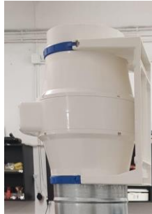
Fig. 16 The fan for extracting the filtered air from the surface of the liquid in the water tank
