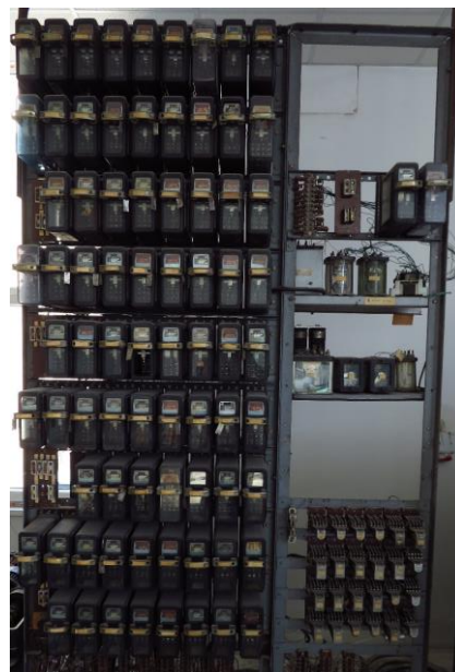
Figure 13. The TET department's relay rack
