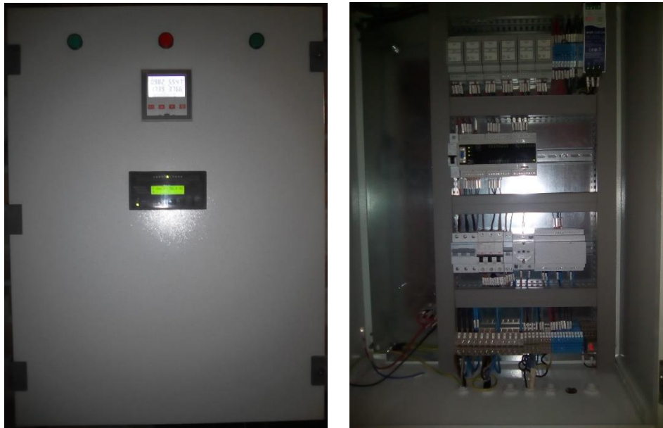
Fig. 18. Control panel and voltage adjustment
