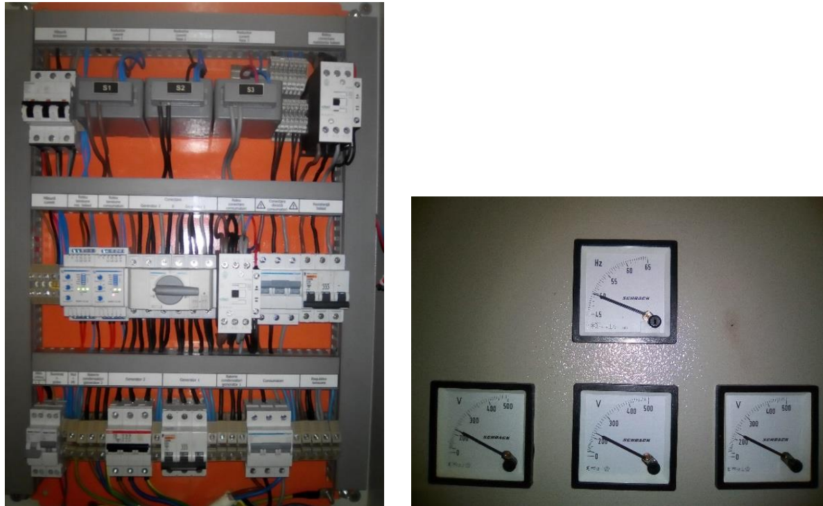
Fig. 15. Microhydropower power supply panel
