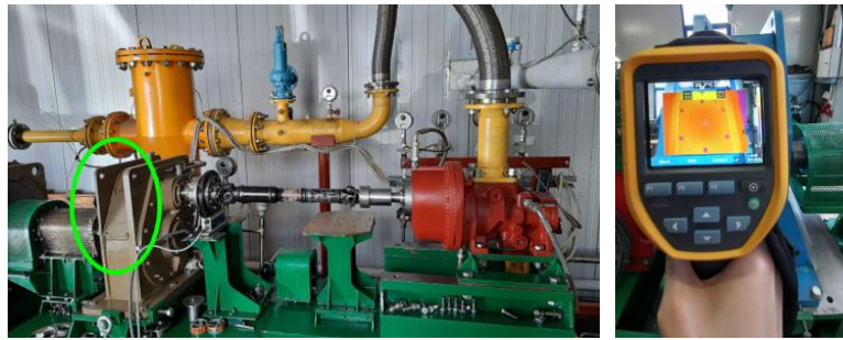
Figure 8. Screw mounting spot for thermoelectric generators and thermal scanning of gearbox cover
