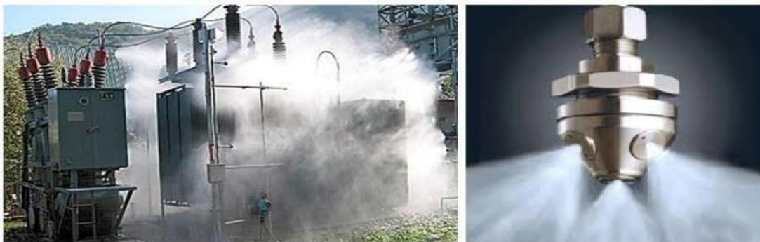
Fig. 18. Fixed extinguishing system with water mist in action and spray nozzle.
