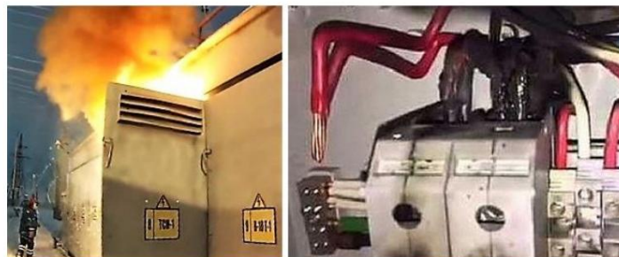
Fig. 3. Fires at electrical panels
