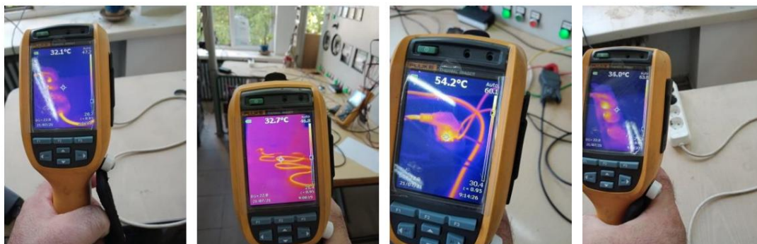
Fig. 15 Temperature difference along the length and at the contact points of the electrical conductor after increasing the load to 12.84 A.
